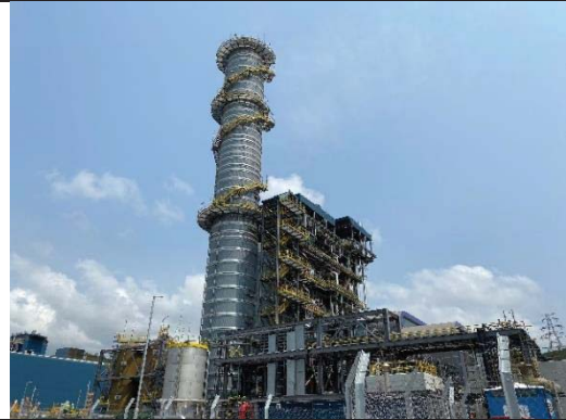
Exhaust Stack of CCGT Unit No.1
